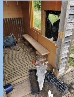
Vandalised shed at Worcestershire Community Land Cooperative allotments
